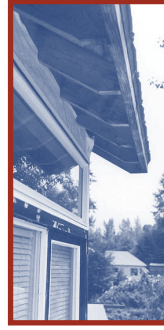
Open eaves, vents not screened (6 pts)
